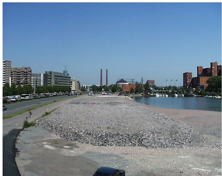
Figure 4. a) Dredging and building of the edge embankment. b) Mass stabilisation work and construction of the compaction layer. c) Preload embankment. Sörnäinen, Helsinki.
